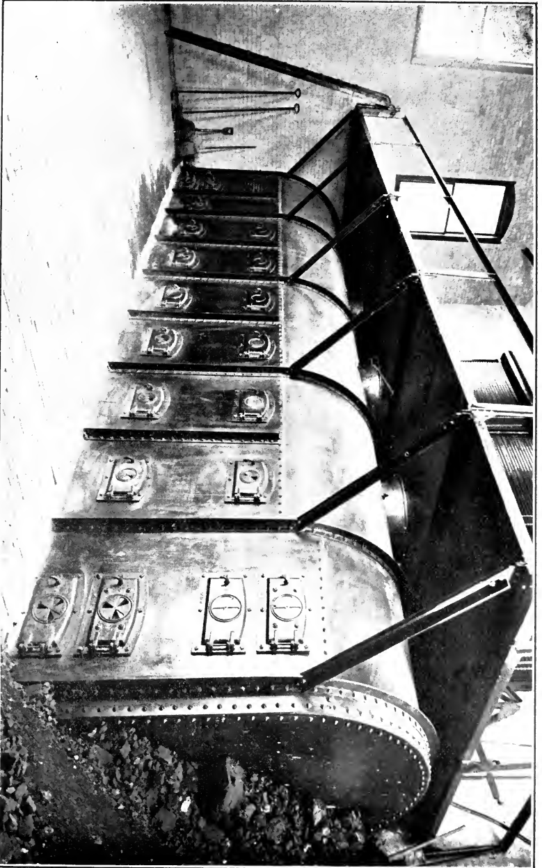
Fig. 20.—Exterior View of Dixon Furnace.
